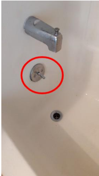
Drain stopper not operable
