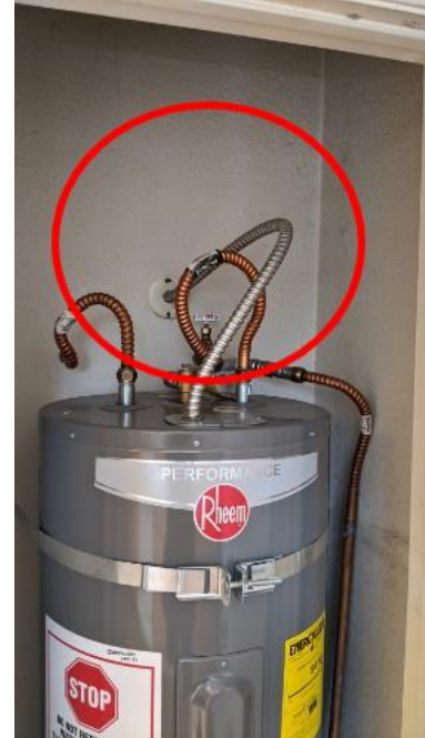
No expansion tank
