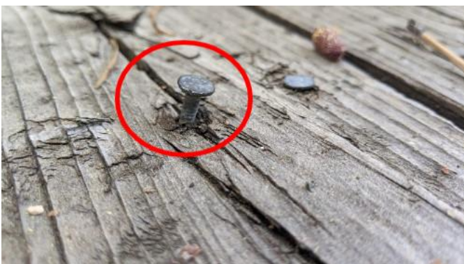
Exposed nails on deck floor surface
