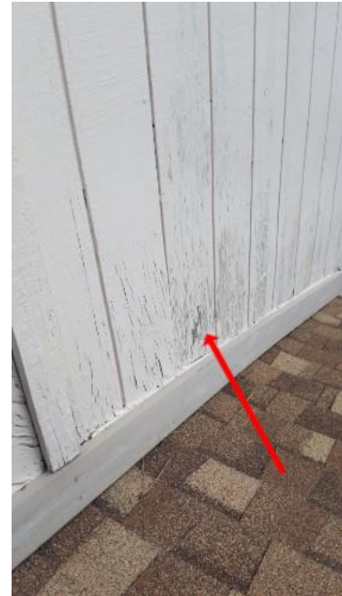
Paint cracking and deterioration on siding above garage(South side of home)
