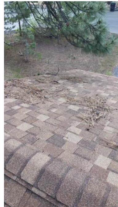
Pine needles/debris on roof
