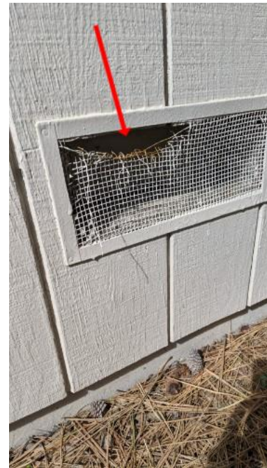
Crawlspace vent damaged
