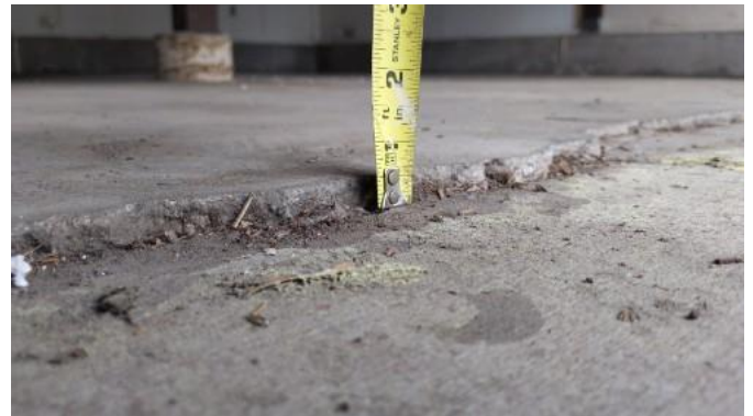
Garage floor crack raised 1/2"
