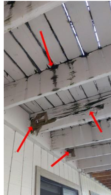
Paint peeling and deterioration under the deck
