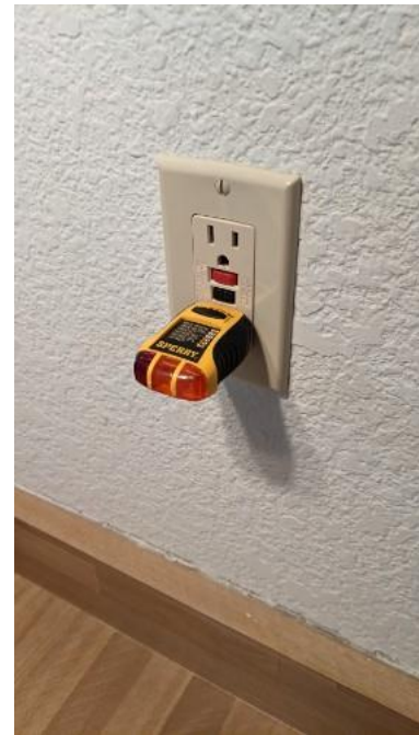
No power to outlet in upstairs bathroom
