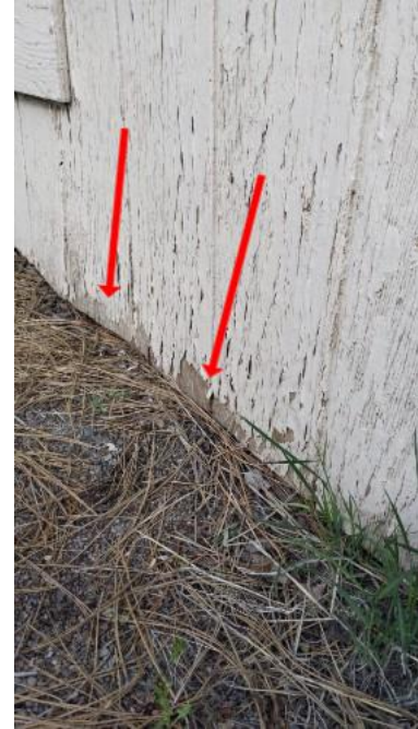
Paint peeling and deterioration
