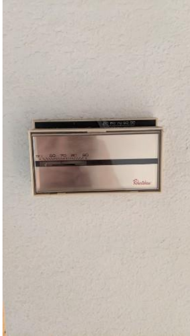
2nd floor thermostat - not working
