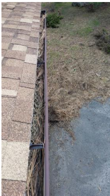
Gutter filled with debris
