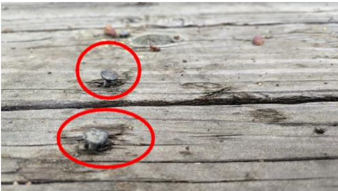
Exposed nails on deck floor surface
