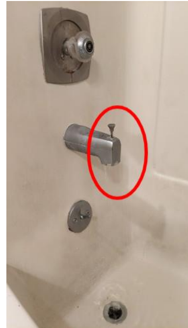
Shower diverter leaking when engaged
