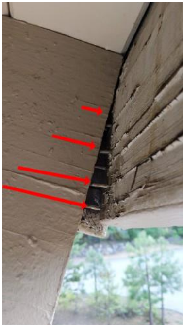
Fascia not secured
