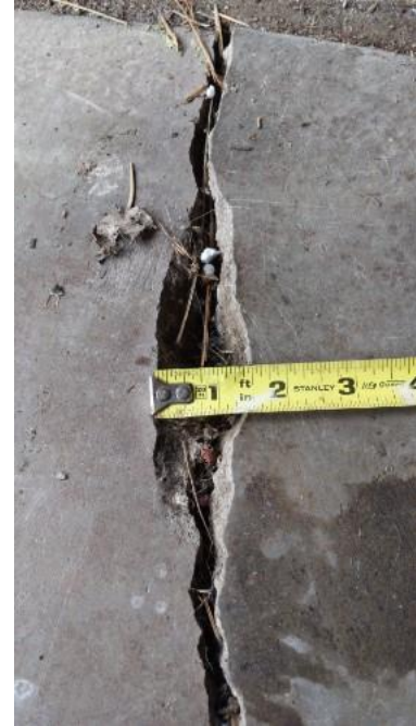
Largest crack in garge has 1 and 1/2" gap
