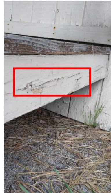
Paint chipping and deterioration
