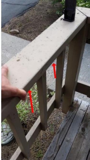
The top part of the railing is loose
