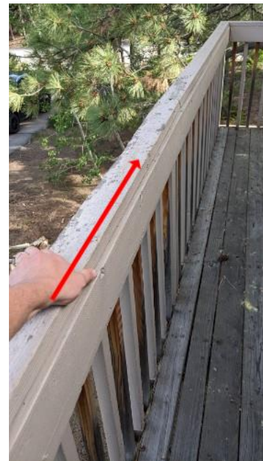
Back deck railing was loose
