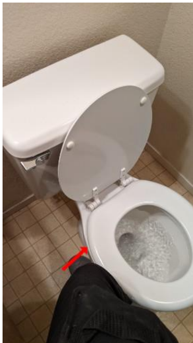
Toilet was loose
