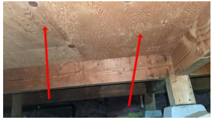
No insulation under flooring
