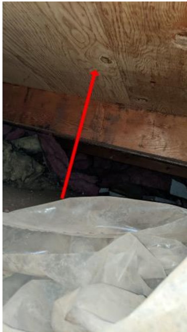
No insulation under flooring
