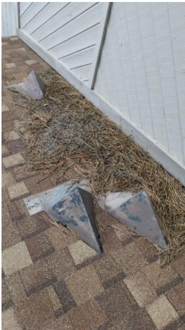
Pine needles/debris on roof
