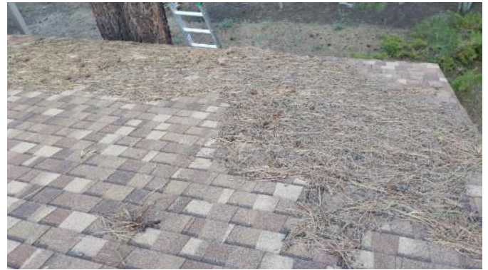
Pine needles/debris on roof
