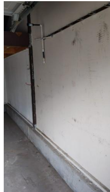
General scuff marks on garge wall
