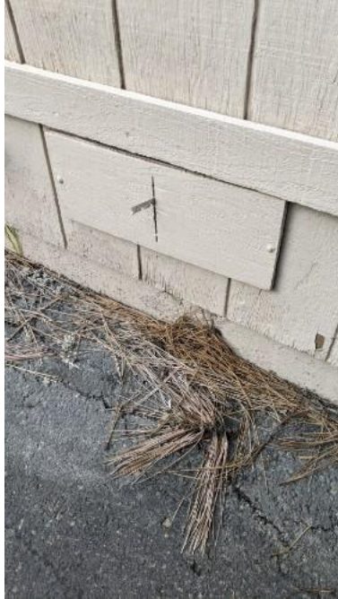
Crawlspace vents sealed up - no ventilation
