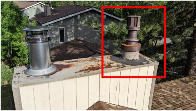
Right is your chimney, left is neighbors. Rust and corrosion observed
