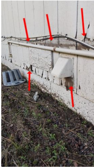
Paint peeling and deterioration on East side of home
