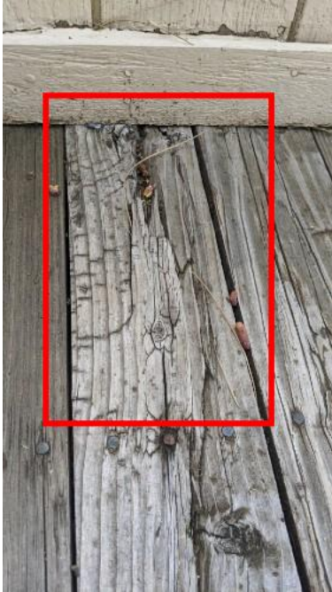
Weathered deck board cracking
