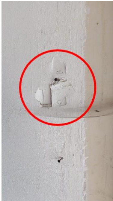
Puncture in the garage wall
