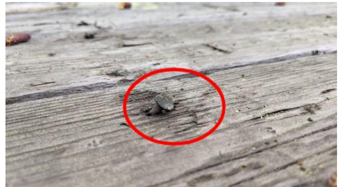
Exposed nails on deck floor surface
