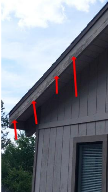
Fascia paint is deteriorating
