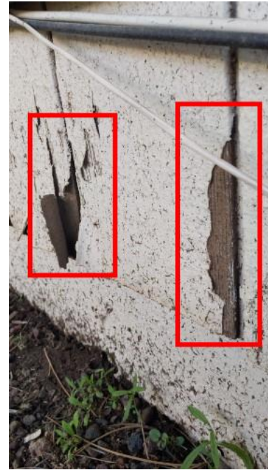
Paint peeling and deterioration exposed wood siding
