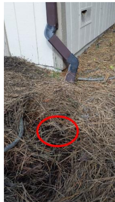
End of gutter is covered and is too close to house
