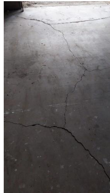
Cracks in garage floor
