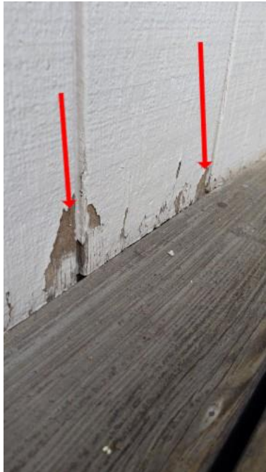
Paint peeling on siding
