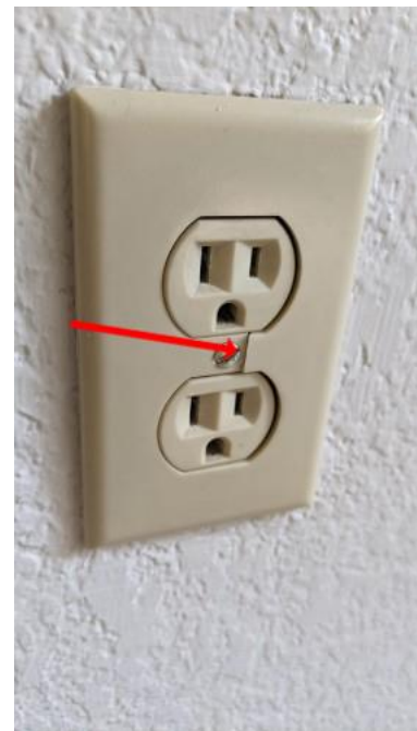
Cracked cover plate
