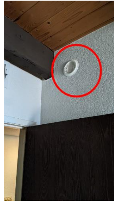
Southeast corner BR - no smoke detector
