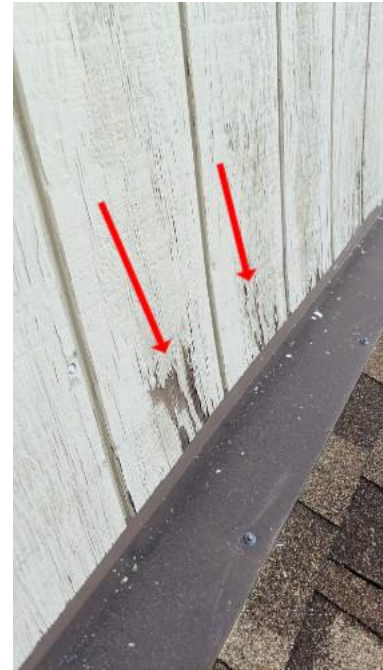
Paint peeling/deterioration on chimney siding
