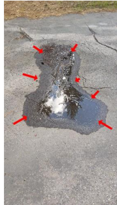
Ponding in driveway
