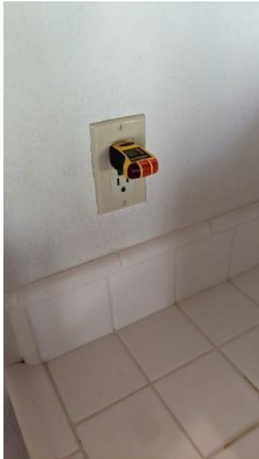
No power to this outlet by wet bar
