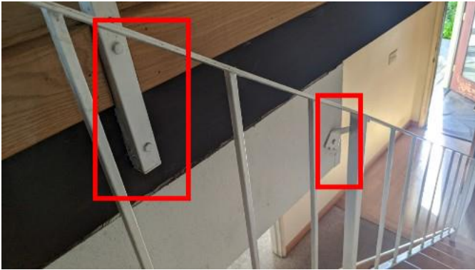
These bolts were loose
