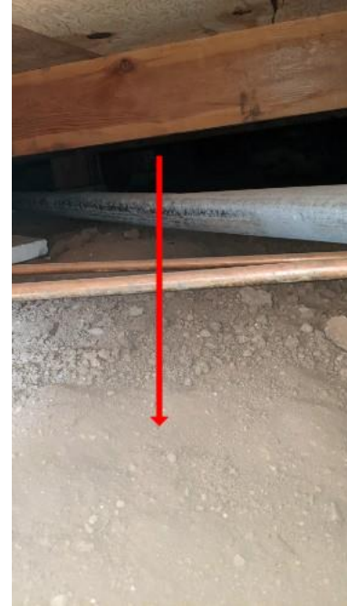
Bare ground - no vapor barrier installed
