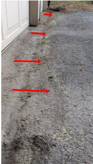
Bulge in the driveway by the garage
