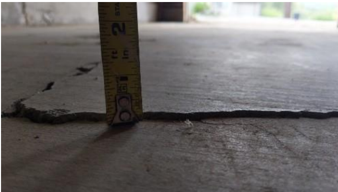
Settlement - near 1/4" height in crack
