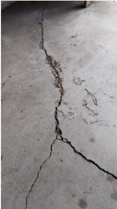
Crack in garage floor
