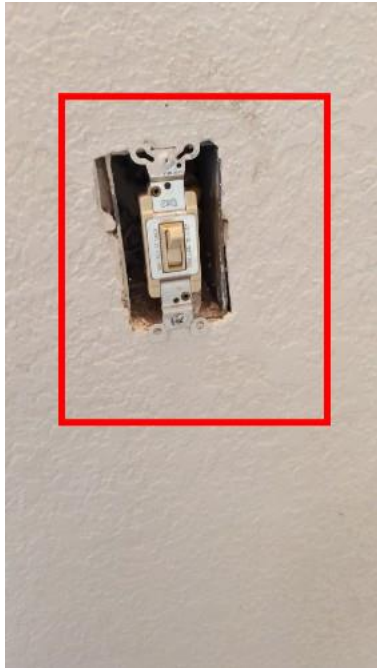
No cover plate - 1st floor by stairway
