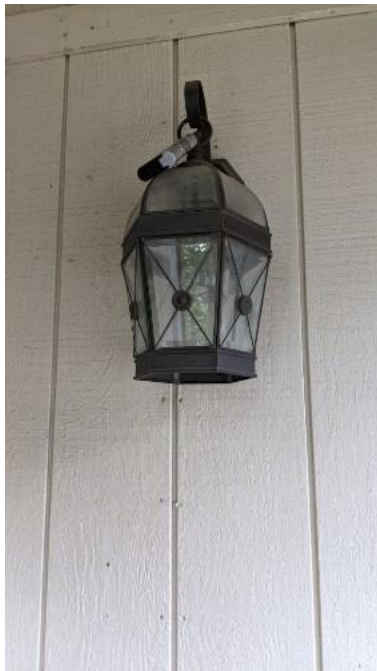
Front entrance light not operating
