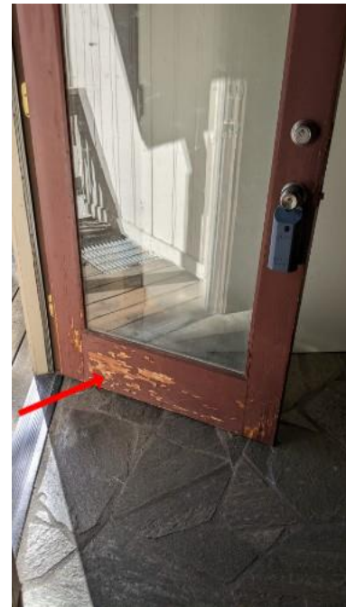
Scuffs and deterioration on front door
