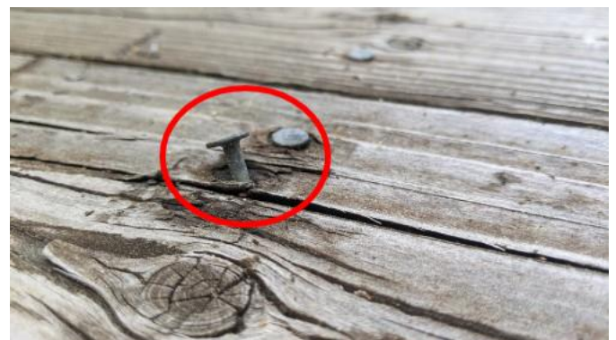
Exposed nails on deck floor surface
