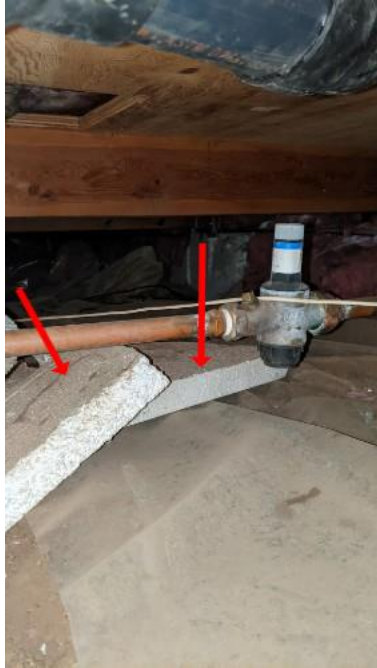
Falling foam board insulation
