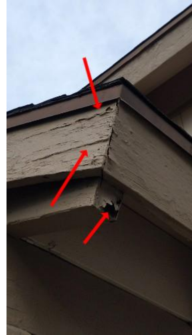
Fascia paint deterioration
