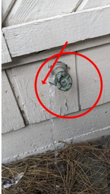
This faucet was working but not properly attached
