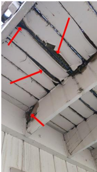
Paint peeling and deterioration under the deck
