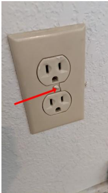
Cracked cover plate
