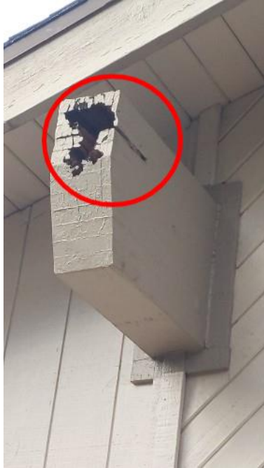
Wood beam deterioration
