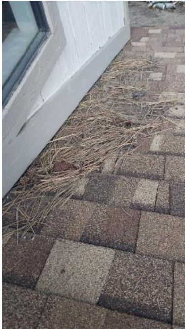
Pine needles/debris on roof
