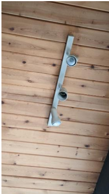
No power to ceiling lights on 2nd floor
