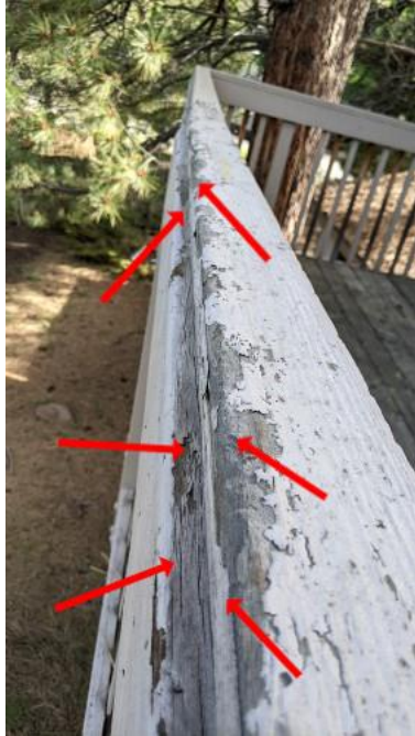
Paint peeling and deterioration on deck railing
