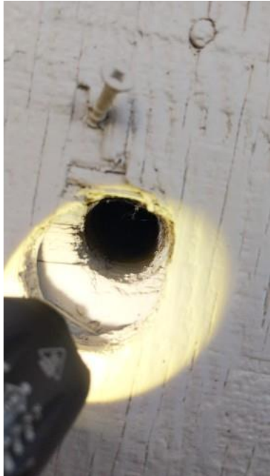
Exposed hole in siding (East side of home)
