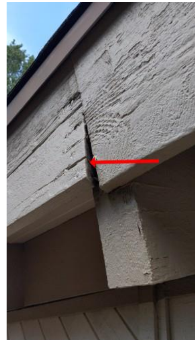
View of fascia not secure from other side
