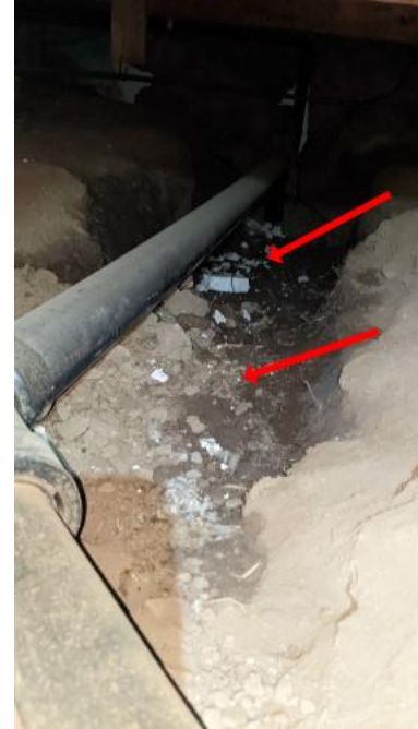
Another view of wet/damp area under drain pipe
