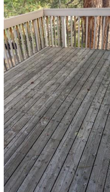
Deck surface weathered
