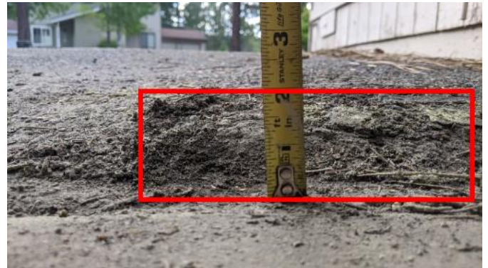
Trip hazard on the corner of the driveway and garage.
