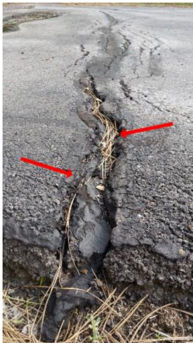
Large crack on side of driveway
