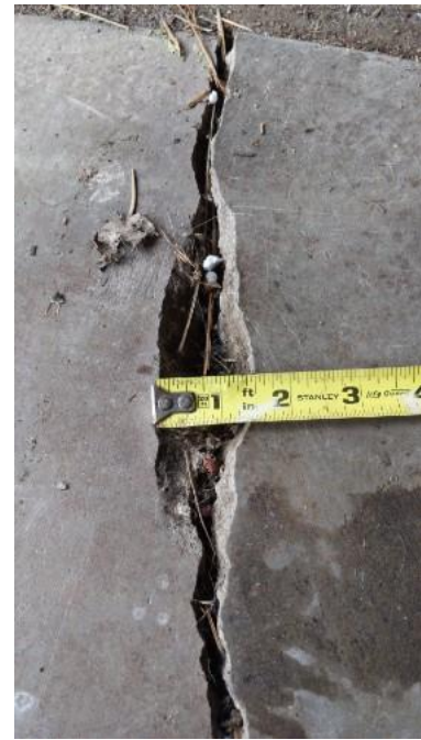
Largest crack in garge has 1 and 1/2" gap
