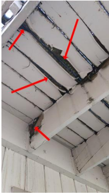
Paint peeling and deterioration under the deck
