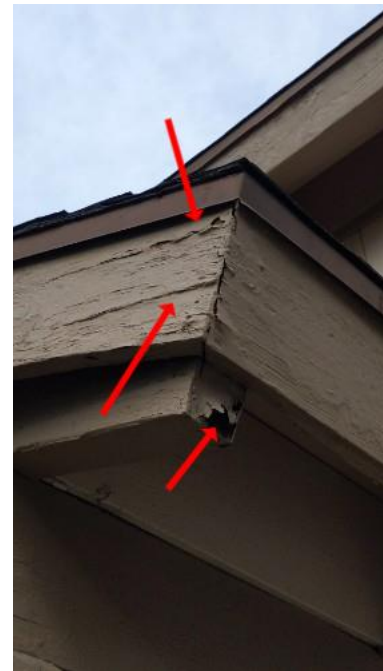
Fascia paint deterioration
