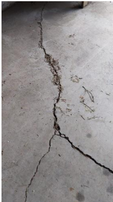
Crack in garage floor
