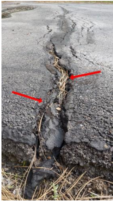
Large crack on side of driveway
