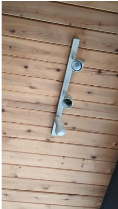
No power to ceiling lights on 2nd floor
