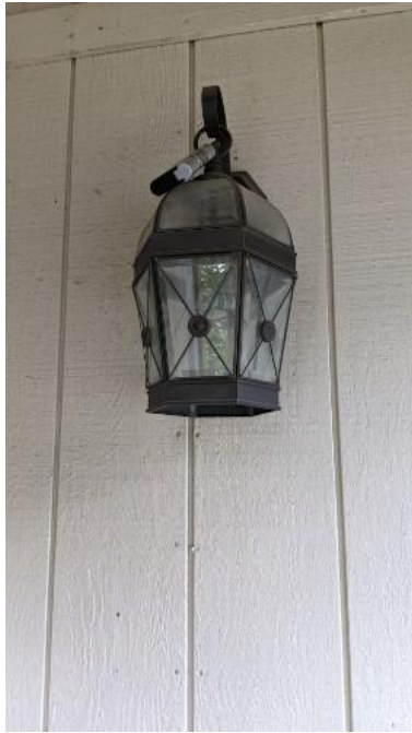
Front entrance light not operating
