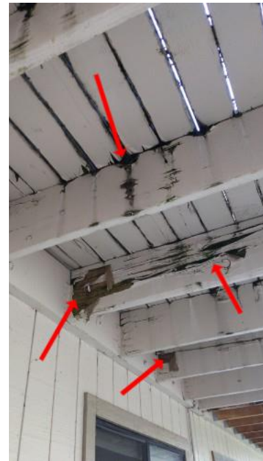
Paint peeling and deterioration under the deck
