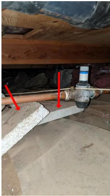
Falling foam board insulation
