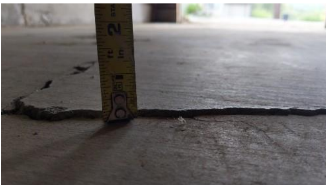
Settlement - near 1/4" height in crack
