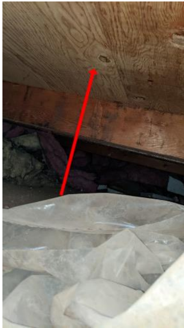
No insulation under flooring
