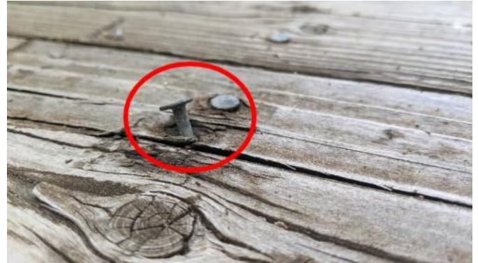
Exposed nails on deck floor surface
