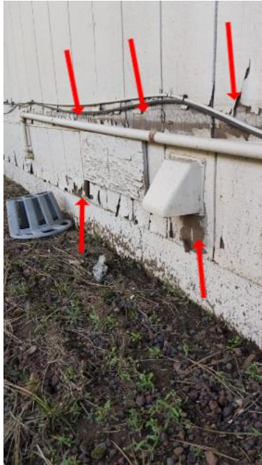
Paint peeling and deterioration on East side of home
