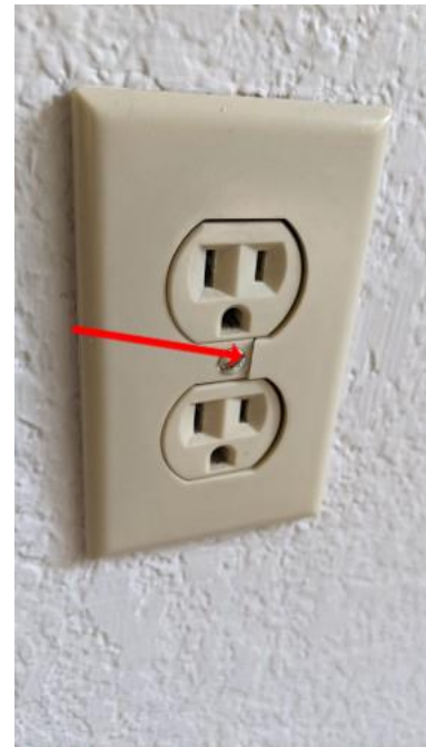
Cracked cover plate
