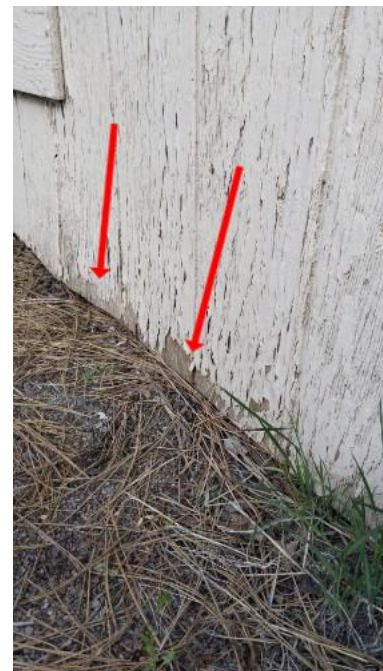
Paint peeling and deterioration
