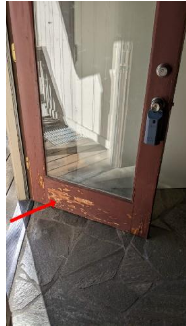
Scuffs and deterioration on front door
