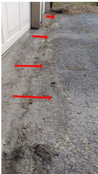
Bulge in the driveway by the garage
