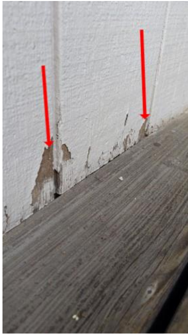
Paint peeling on siding
