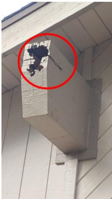
Wood beam deterioration
