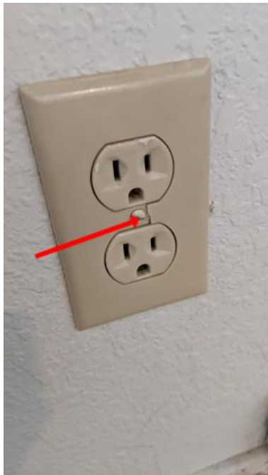
Cracked cover plate
