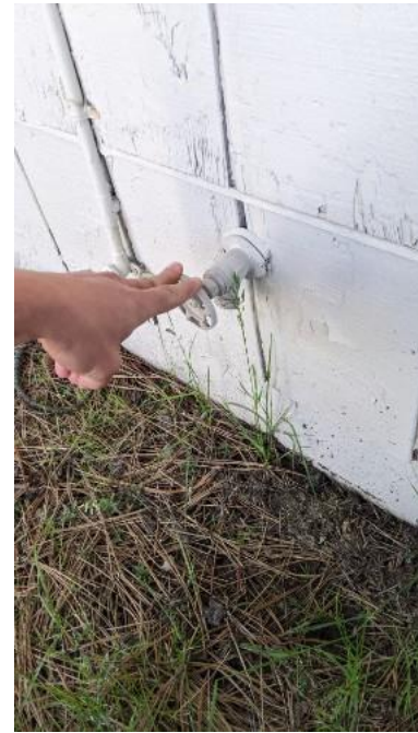
Faucet on back of home (East) not working
