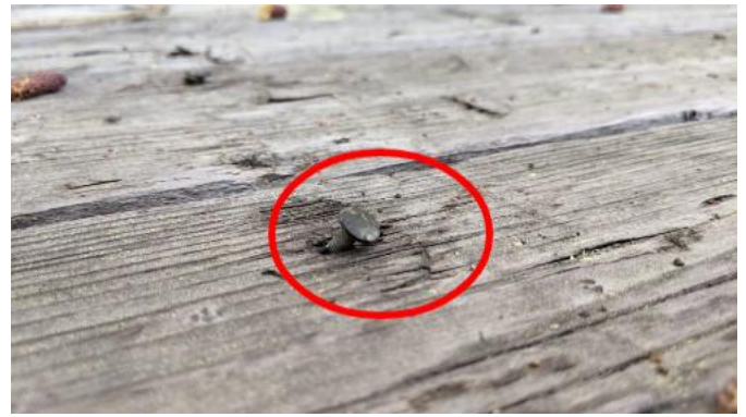
Exposed nails on deck floor surface
