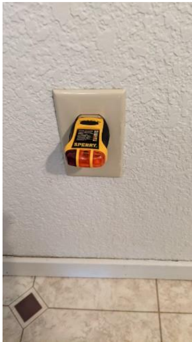
No power to outlet in upstairs bathroom
