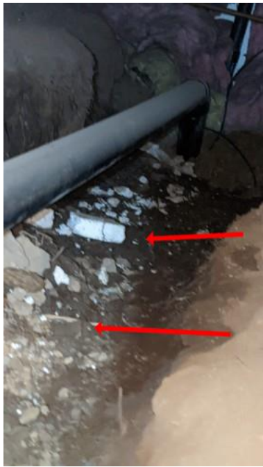
Wet/damp area under drain pipe and soil is lower
