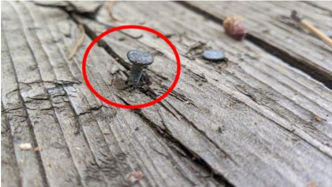
Exposed nails on deck floor surface
