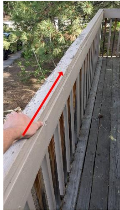
Back deck railing was loose
