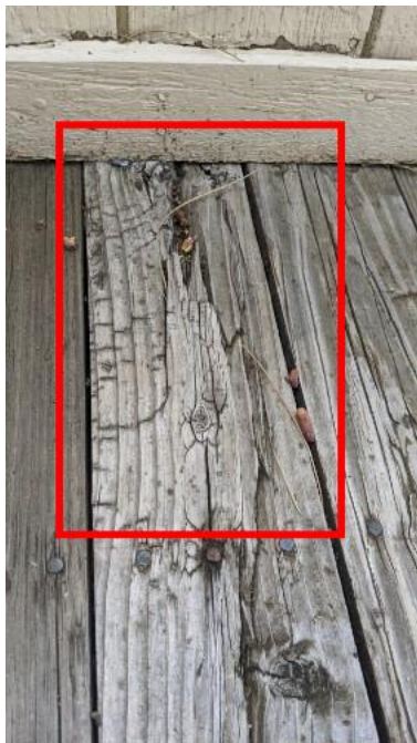
Weathered deck board cracking
