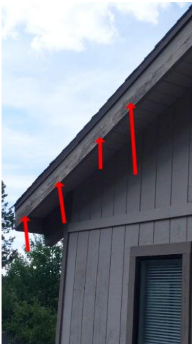
Fascia paint is deteriorating
