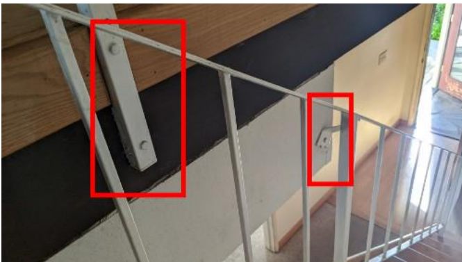
These bolts were loose
