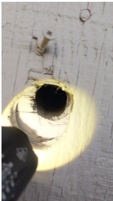
Exposed hole in siding (East side of home)
