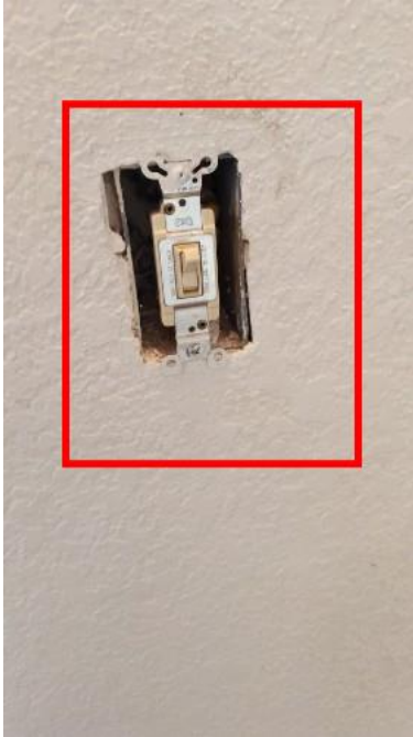
No cover plate - 1st floor by stairway
