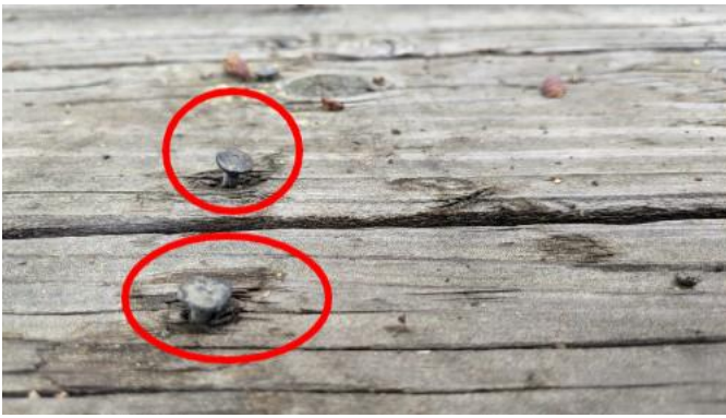
Exposed nails on deck floor surface
