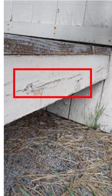
Paint chipping and deterioration
