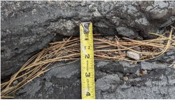
2" gap measured in the crack on side of driveway
