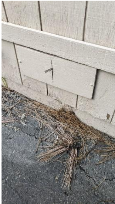
Crawlspace vents sealed up - no ventilation
