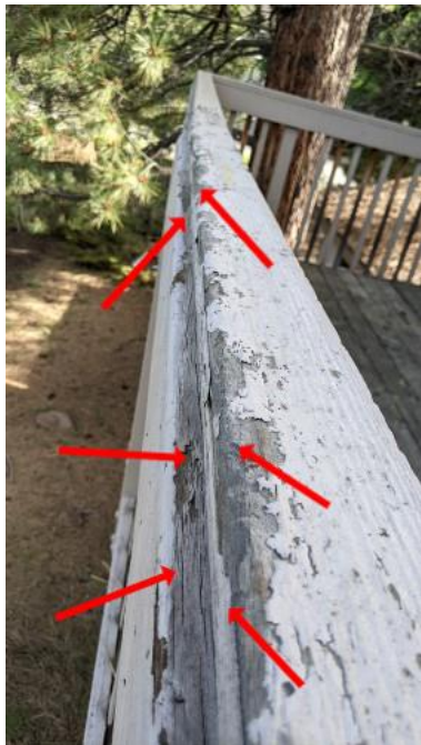
Paint peeling and deterioration on deck railing
