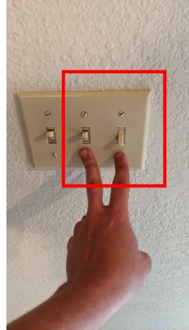
These two switches by front door did not operate
