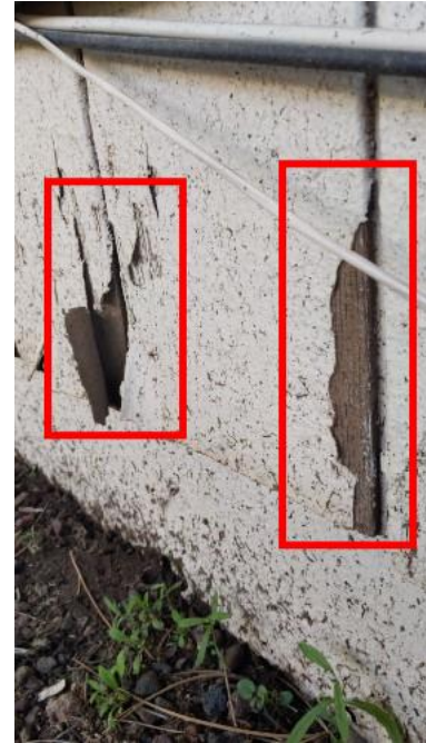
Paint peeling and deterioration exposed wood siding
