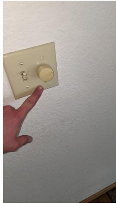
Control to ceiling lights on 2nd floor not working
