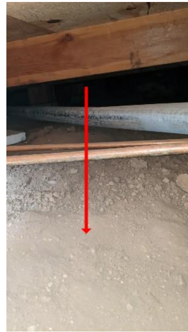
Bare ground - no vapor barrier installed
