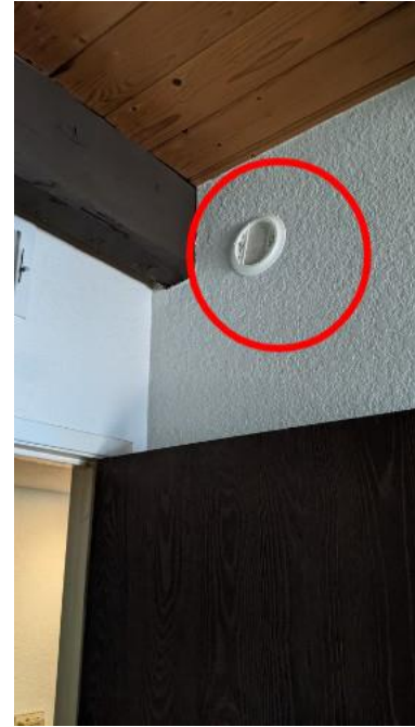
Southeast corner BR - no smoke detector
