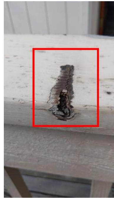
Deterioration on railing
