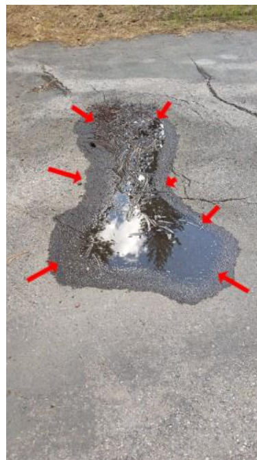
Ponding in driveway
