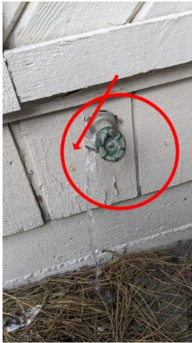
This faucet was working but not properly attached
