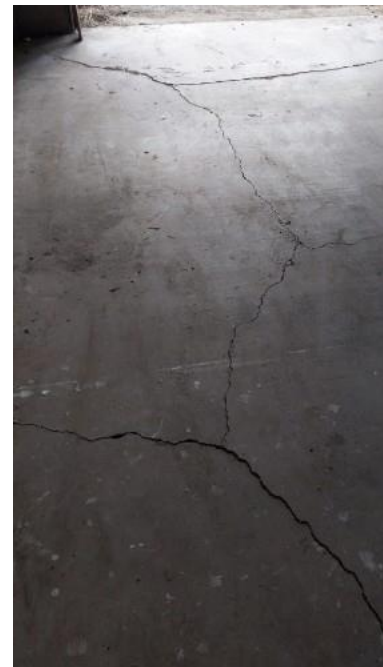
Cracks in garage floor
