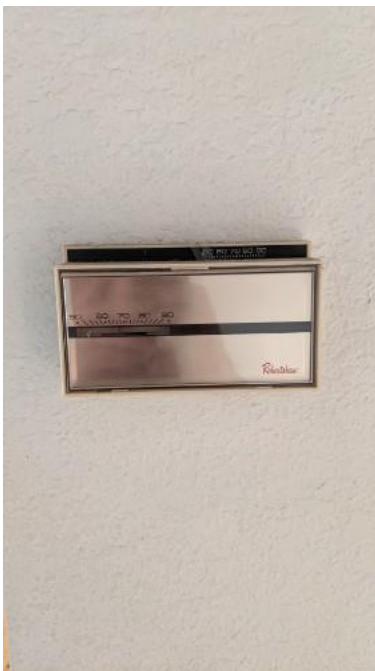
2nd floor thermostat - not working
