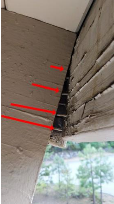
Fascia not secured
