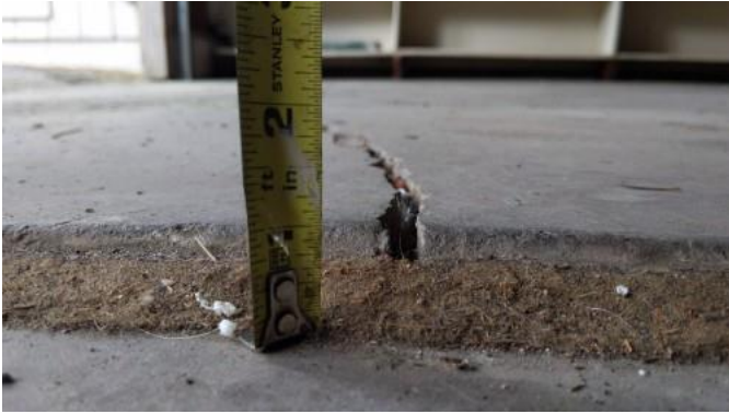
Middle divider of the two car garage is raised nearly an inch
