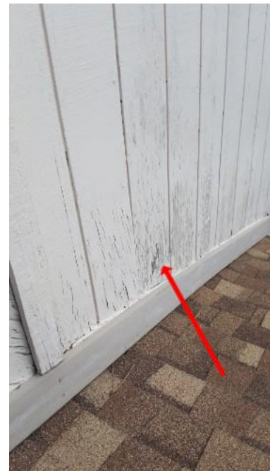
Paint cracking and deterioration on siding above garage (South side of home)
