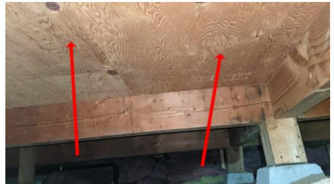
No insulation under flooring
