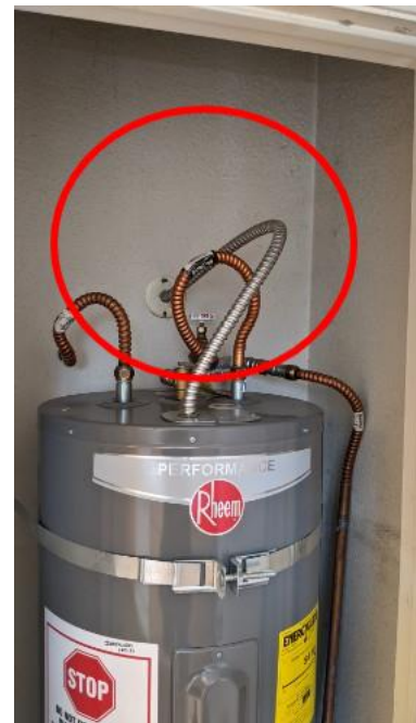
No expansion tank
