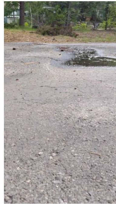
Ground angle of the ponding noting the driveway height differences
