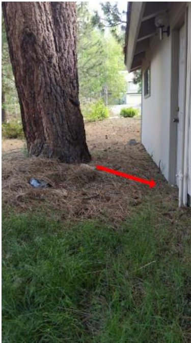
Slopes towards garage access door and East side of home.
